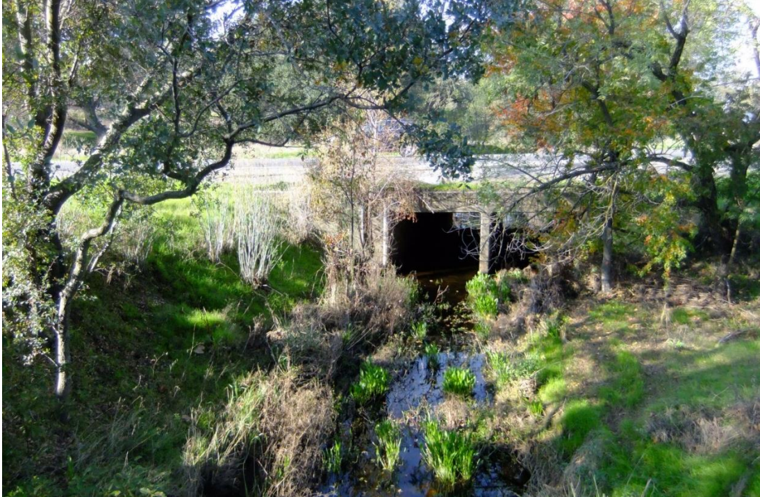
Photo 8. Looking west from the bicycle/pedestrian bridge over SBPGC on the east side of Washington Boulevard, north of the Andora bridge. Photo depicts downstream view of SBPGC and box culvert under roadway. Photo taken November 11, 2016.
