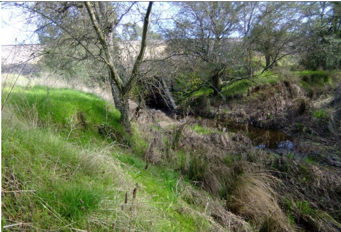
Photo 6. Looking east from City open space preserve at confluence of SBPGC and SVT, and box culvert under existing UPRR track. Culvert is upstream of confluence. Photo taken November 11, 2016.
