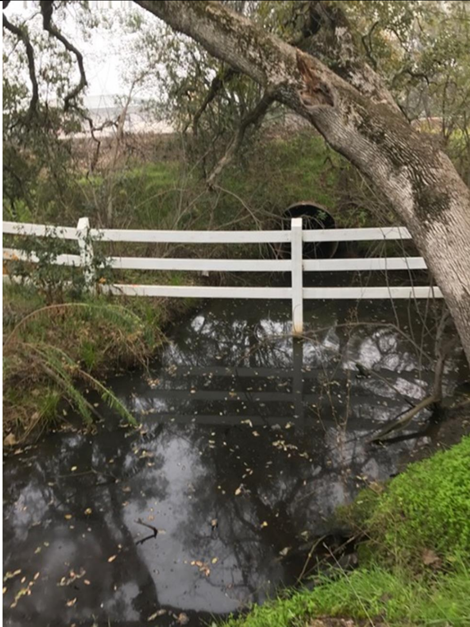
Photo 7. Looking northeast from the west side of Washington Boulevard, south of the Andora bridge, at pipe culvert under the roadway. Photo depicts upstream view of the unnamed tributary. Photo taken December 6, 2016.
